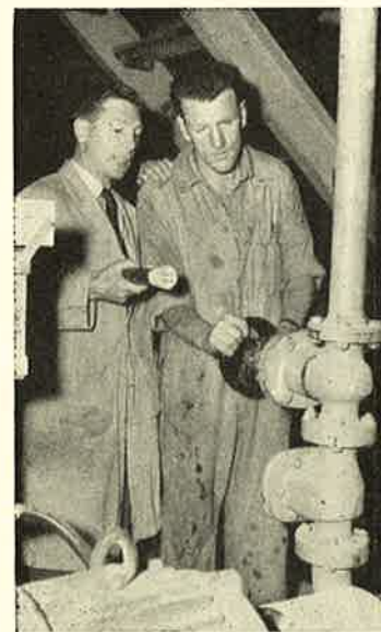
Engineer John Minton discusses water controls with fireman Bill Harkins on the condenser floor.
