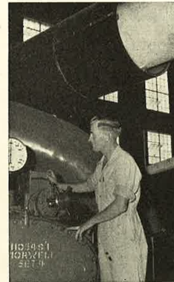
Noel Edmunds, acting turbine driver, at the governors end of the No. 1 low pressure turbine.
