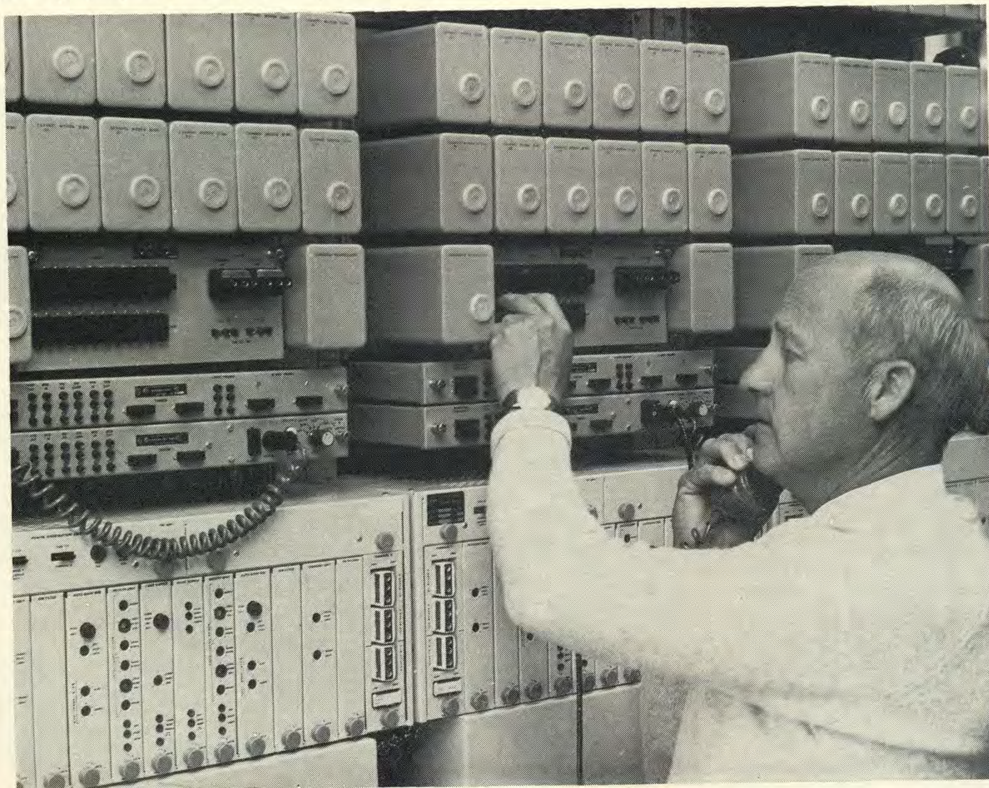
Jack Peacock, Carriers Supervisor, checking traffic on the Yallourn-Morwell Cable Carrier at Yallourn. The equipment rack on his left is the Yallourn-Hazelwood carrier
