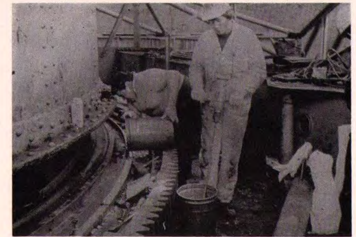
Mixing and pouring epoxy mortar under lower slew race are L/H Fitter Peter Manicola and Apprentice John Ericsson.
