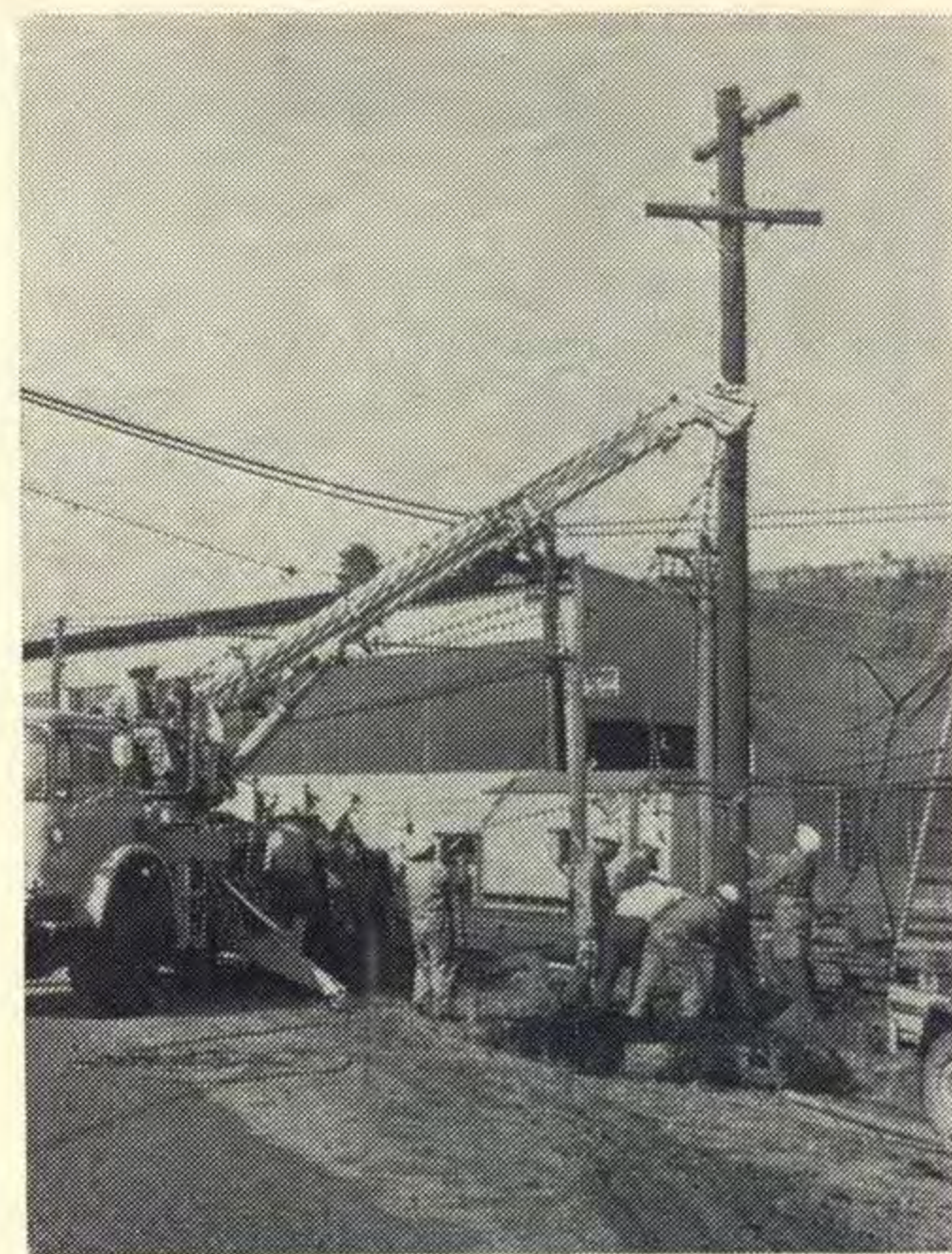
The Proline, at work erecting a pole alongside traction lines, demonstrates its manoeuvrability.
