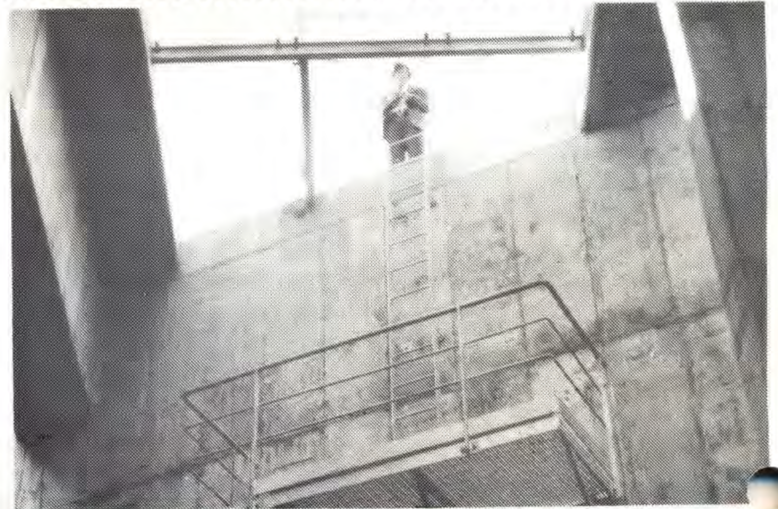
This picture above was taken from the floor inside the station, looking toward its ceiling.
