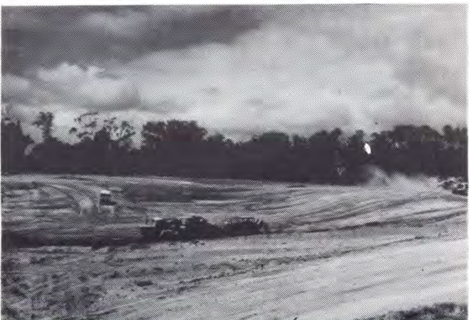
Scrapers and bulldozers are currently working on the earth works for the Loy Yang power station.
