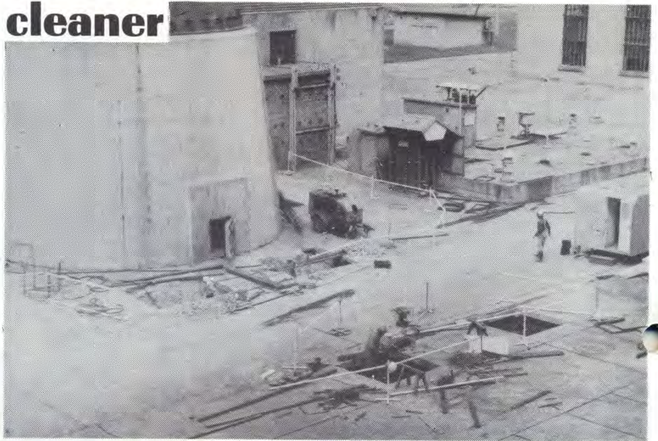
Initial site works (above) have begun for the installation of the electrostatic precipitators at the Morwell Briquetting and Power Installation.
