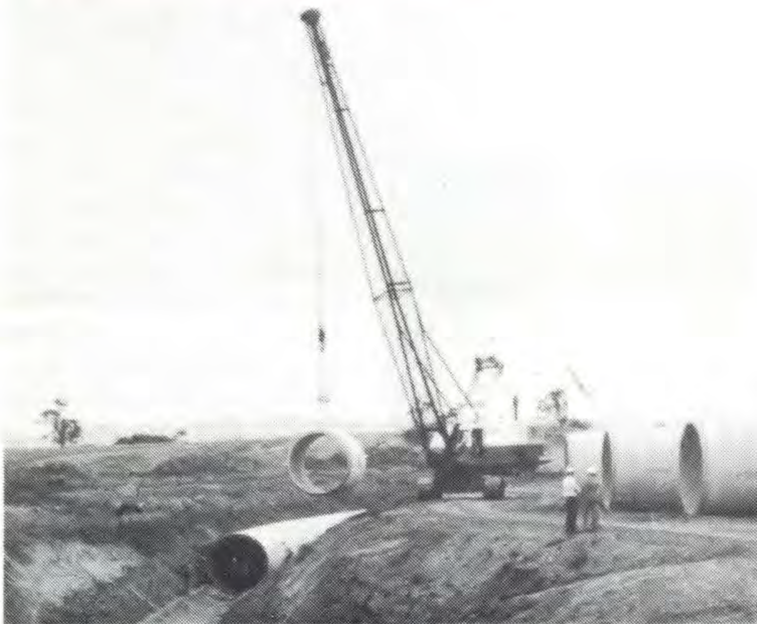
Laying the 13 tonne pipes at the diversion is a major job, this picture gives an excellent overall view of the procedure.
