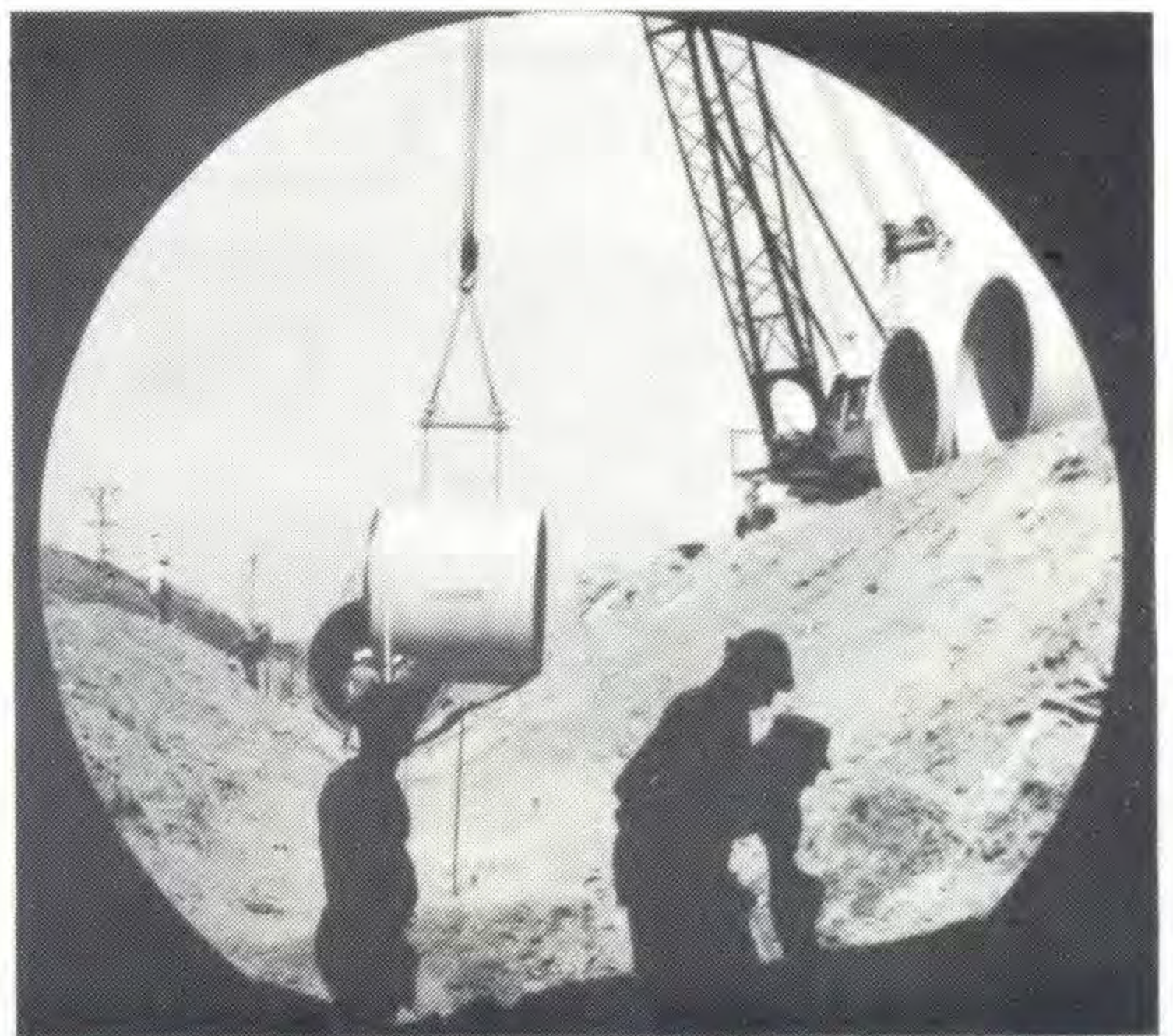
This spectacular picture of pipes being laid was taken from inside one of the 13 tonne pipes.
