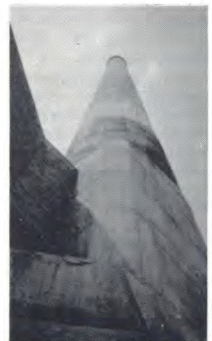
The 328ft concrete stack at the Yallourn Briquette factory had a 40 ft. diameter base.
