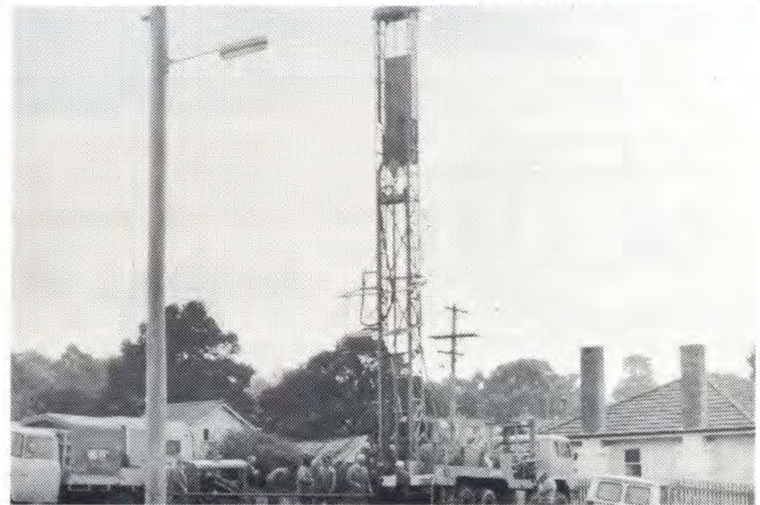
The new drilling rig (above) was pictured earlier this month working in Yallourn.
