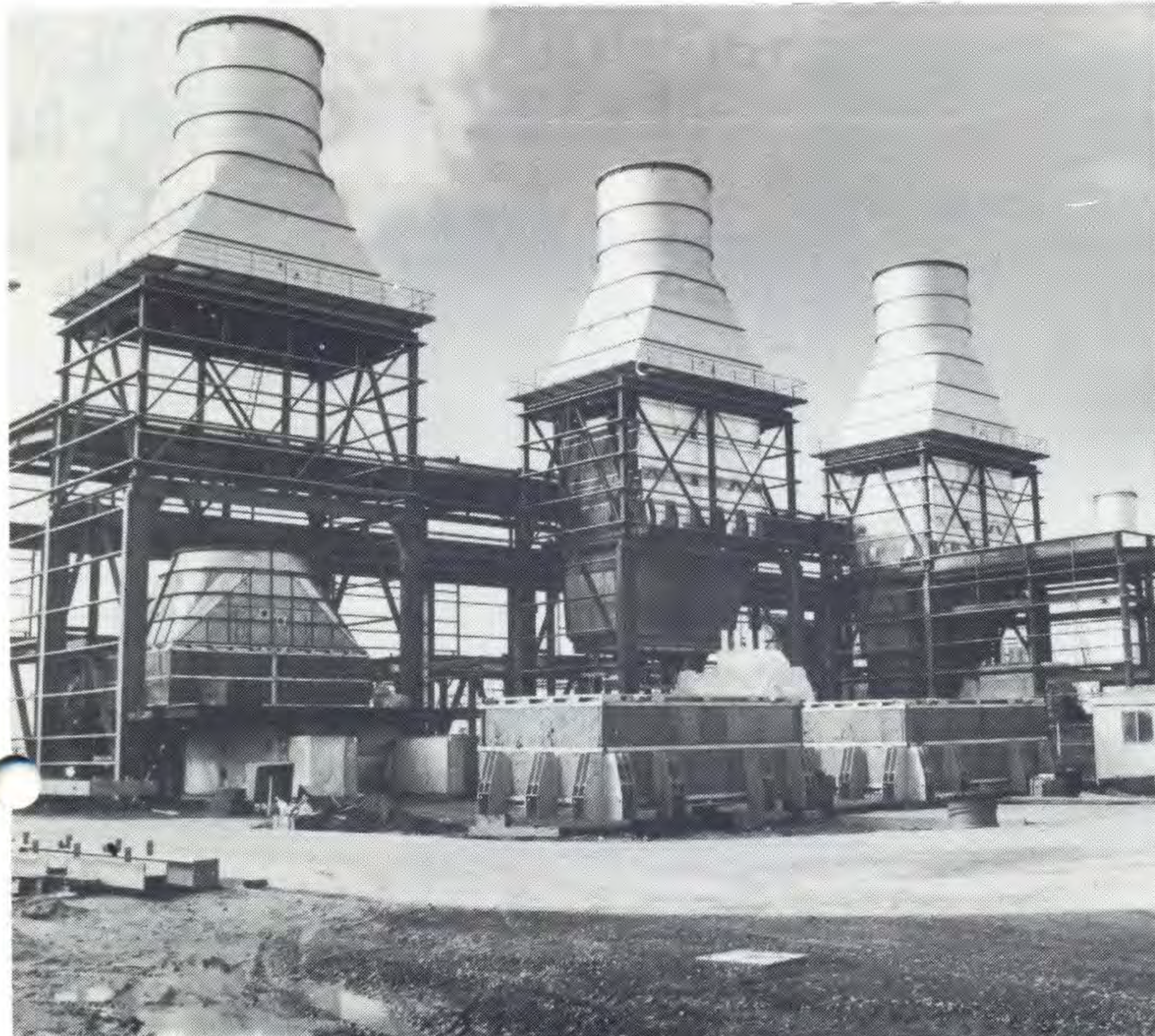
WORKK is progressing steadily on Jeeralang 'B' gas turbine station south of Morwell.
