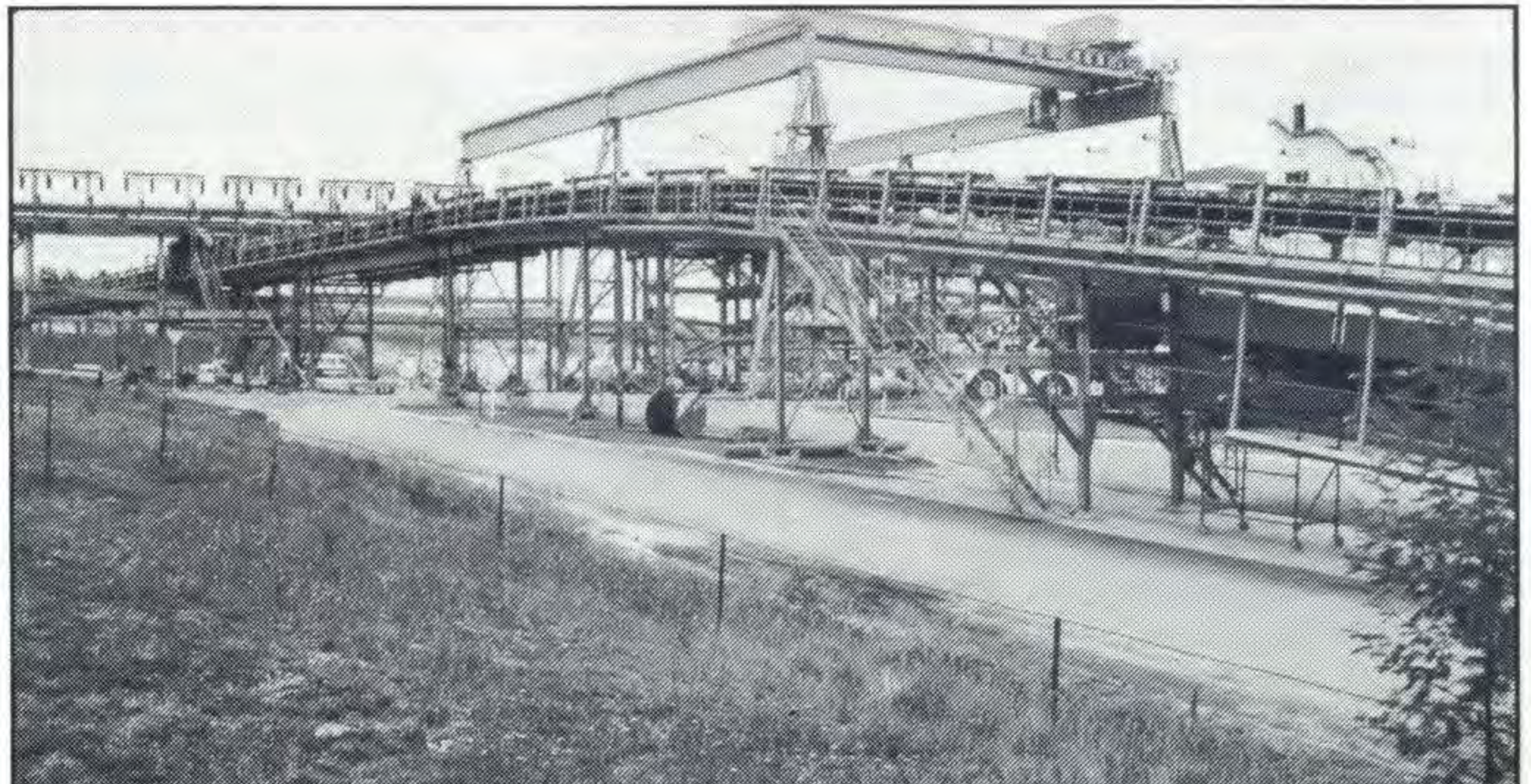
Above: The two metre wide 700 conveyor is almost ready for commissioning with the completion of the no-load run for the belt.
