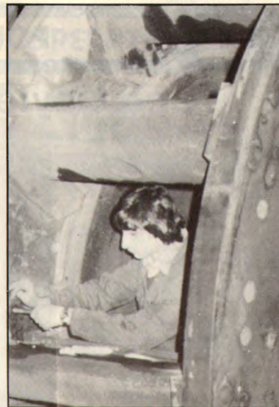
Above: Non-refit work isn't being neglected at the workshops. Here, Bradley Staycho, a third year apprentice fitter is working on a Yallourn W beater wheel.
