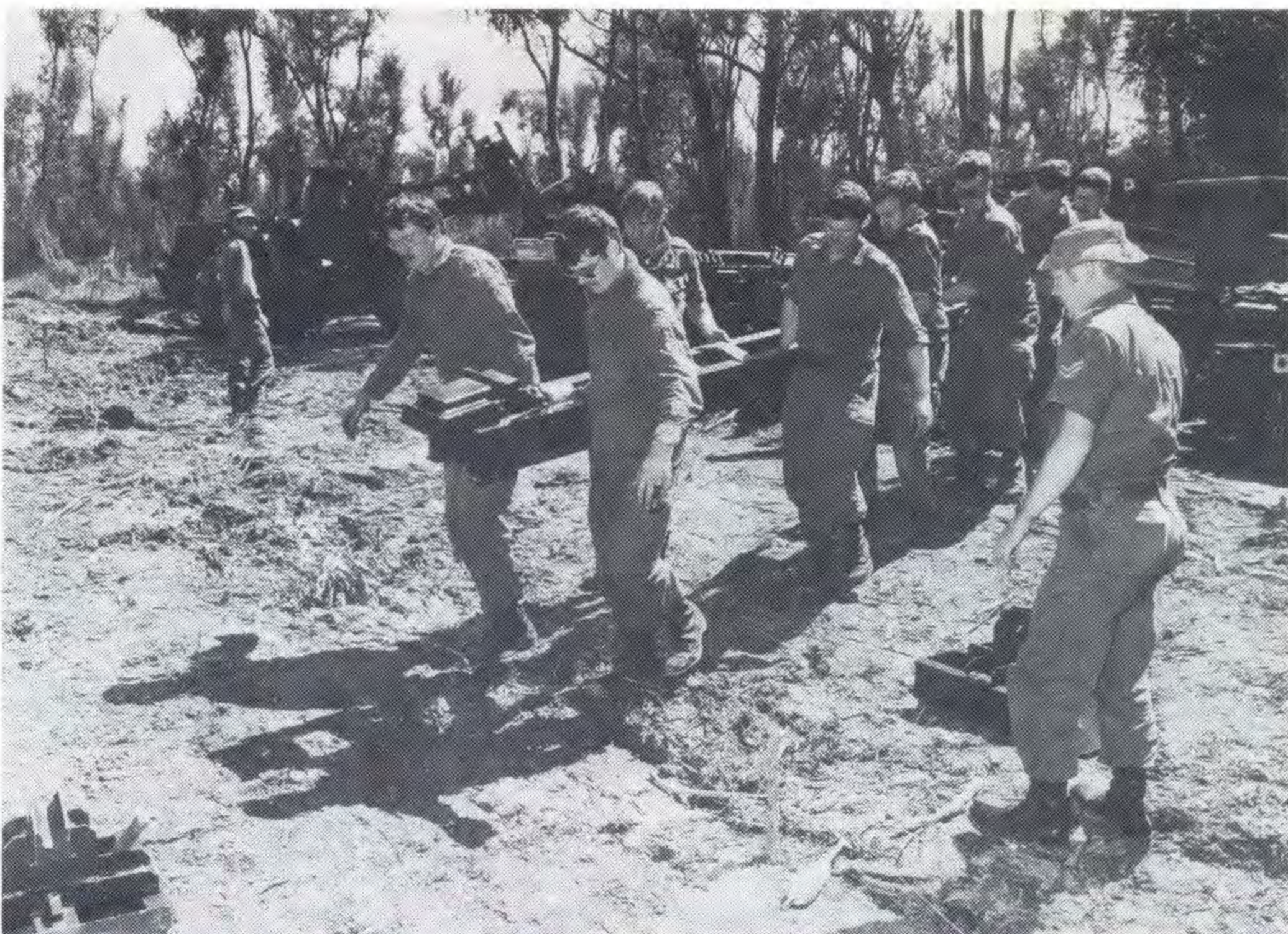
ABOVE: Members of the 38th Field Squadron move a 300 kg bank seat beam into position as part of a bridge building task.
